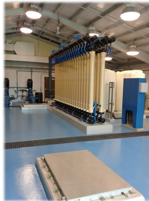
Horn Creek Treatment Equipment
