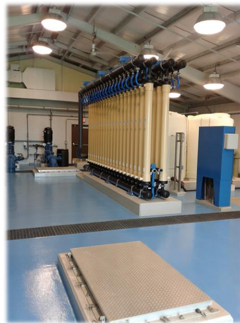
Horn Creek Treatment Equipment
