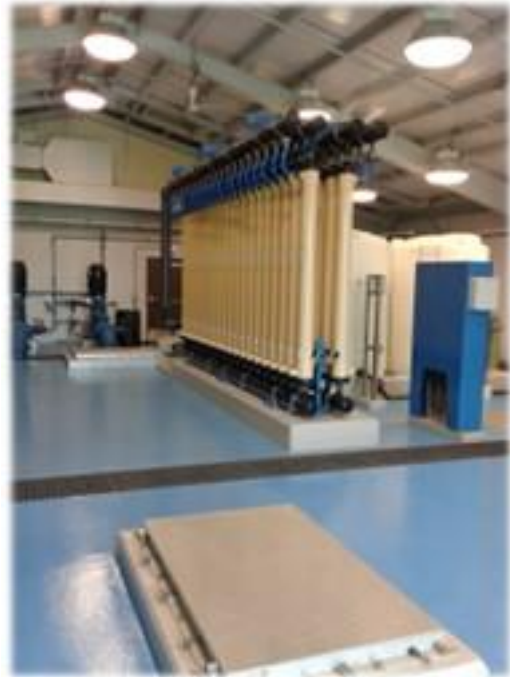
Horn Creek Microfiltration System
